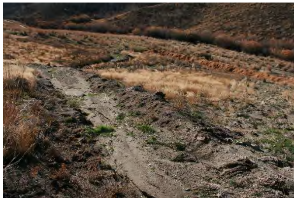
A newly constructed earthen sediment basin with broadcast seed and erosion fabric, prior woody shrub plantings; Cabbage Gulch
