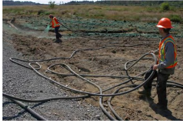
Hydroseeding applications are restricted to roadsides and can extend upwards of 300- 500 feet from pull-out.
