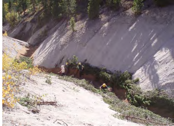
Brush bundles being installed in a large erosion gully in the Mt. Haggin WMA
