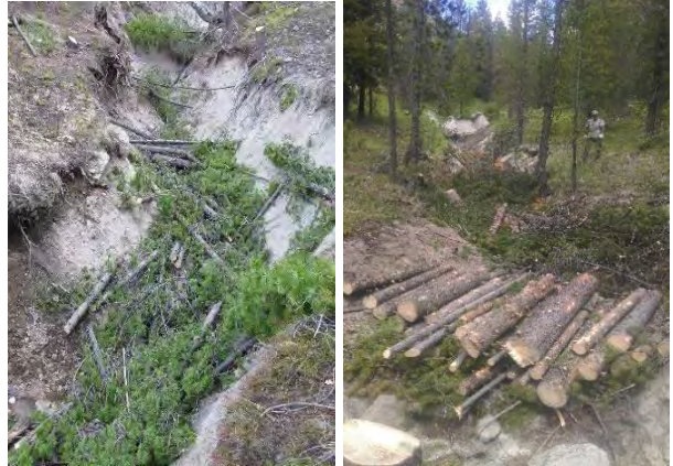
Two examples of slash filters utilizing forest thinning byproducts to capture sediment and fill erosion gullies.
