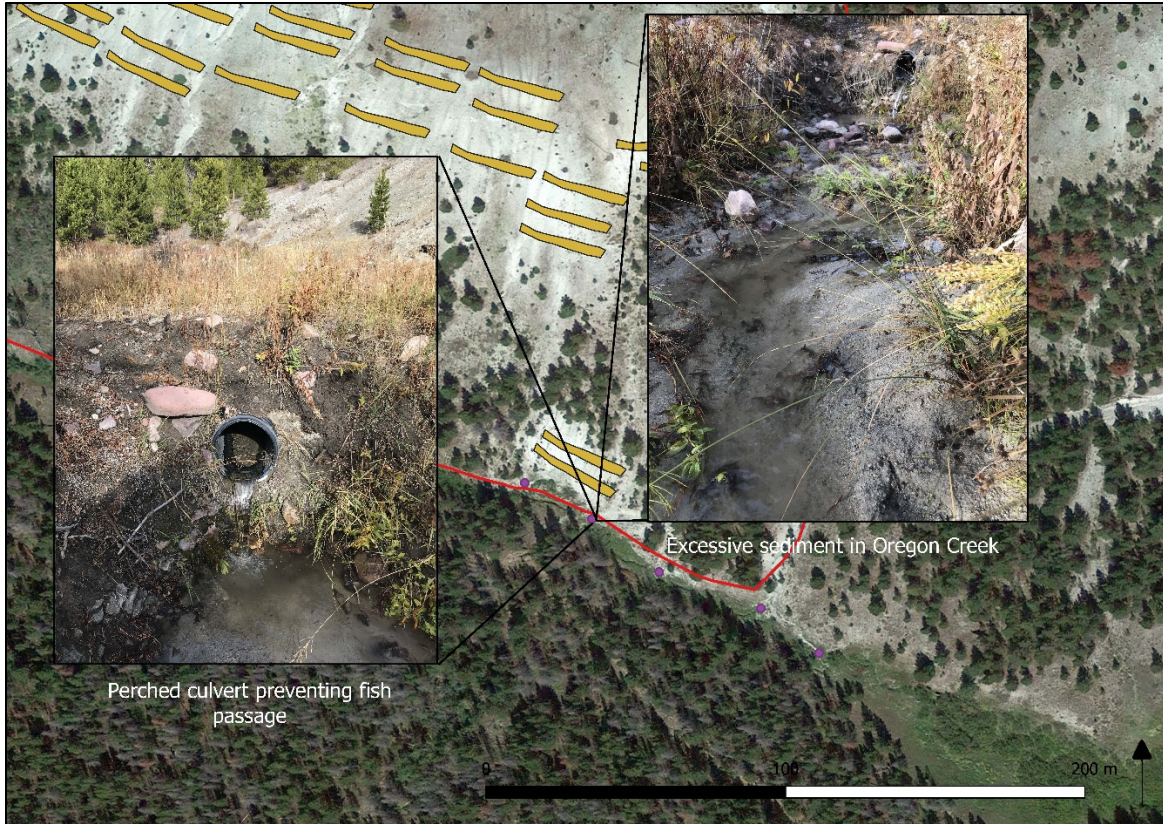
Figure 8. Perched culvert and sediment choked stream in the upper reaches of project area.
