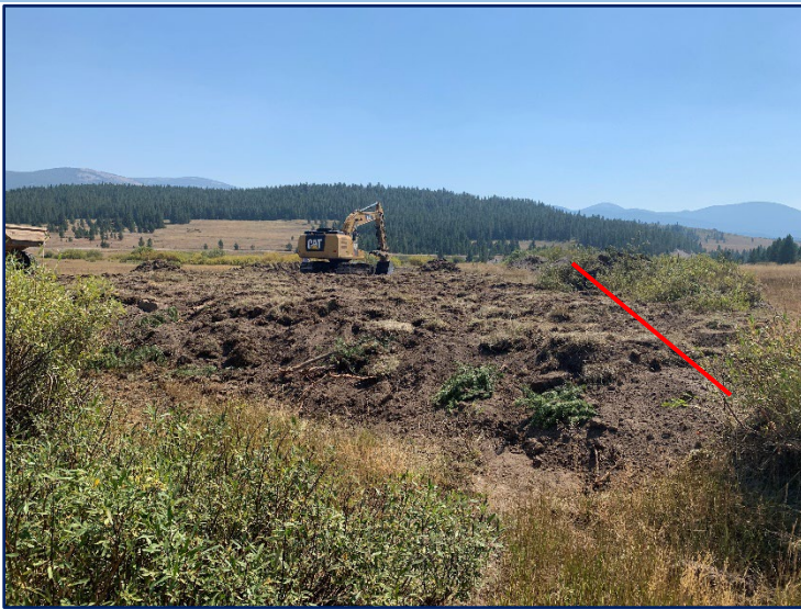
“Stage 0” mid construction (2022). Note: red line signifies where the old channel alignment was.
