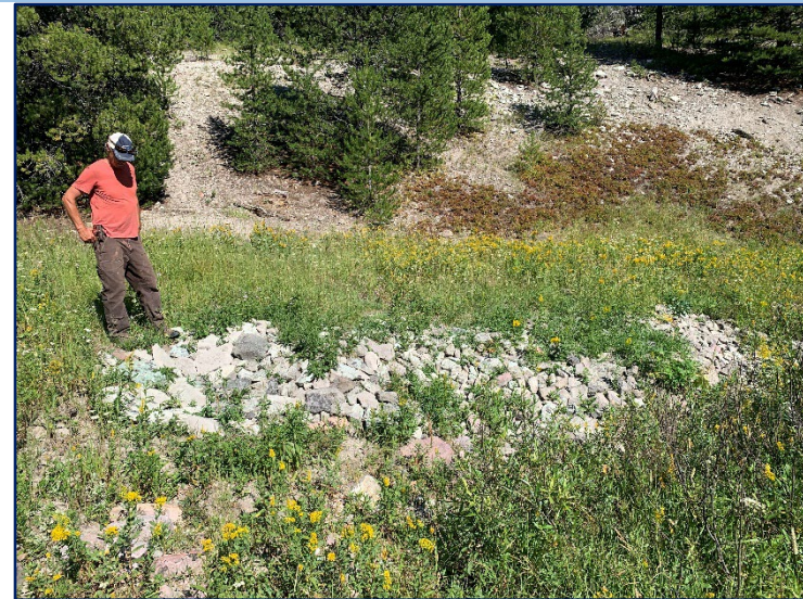
Touring the stream project site with NRDP (2023). Ray Vinkey is inspecting a head cut structure installed in the middle reach in 2022.
