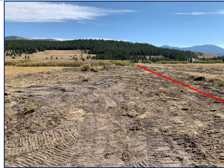
“Stage 0” mid construction (2022). Note: red line signifies where the old channel alignment was..
