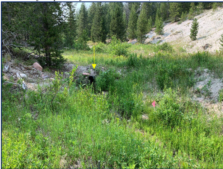
Before photo of perched culvert (2022).
