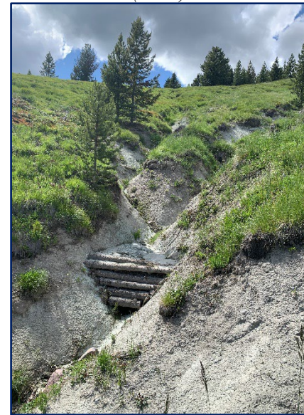
Upper most gully check dam at capacity (2023).
