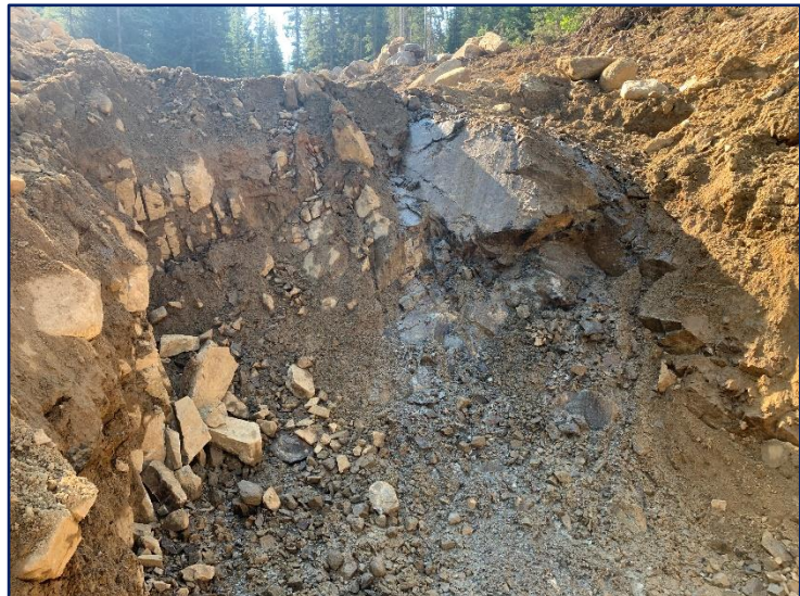
Unexpected impenetrable bedrock layer in the project alignment.
