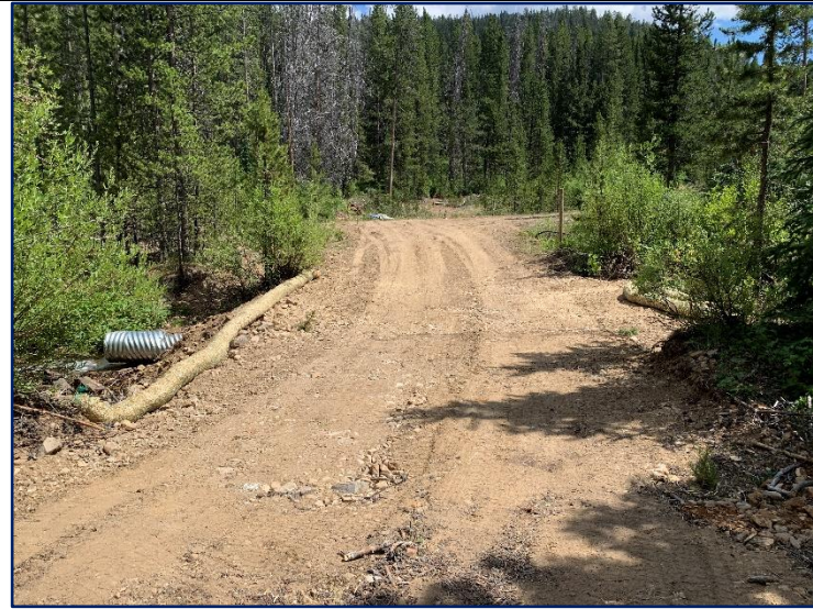
Second stream crossing and straw wattle BMP entering the staging area. Both stream crossings used 18" x 30 corrugated metal pipes.
