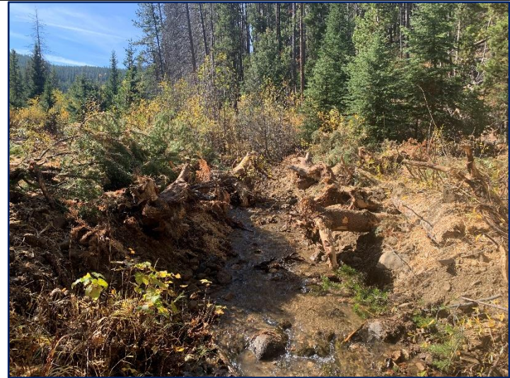
Looking upstream at second eroding bank/stream crossing post-restoration. Note the large root was anchored in to both sides.
