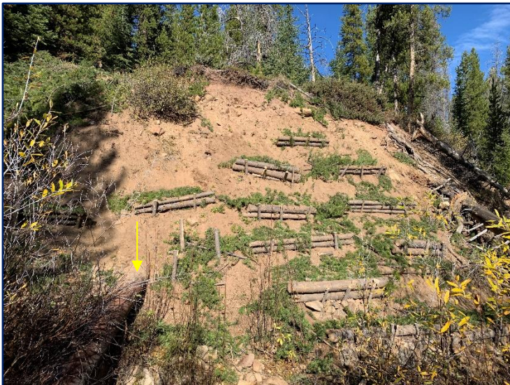
"After" photo of first high and eroding bank post low-tech wattle fence installation. Looking west.
