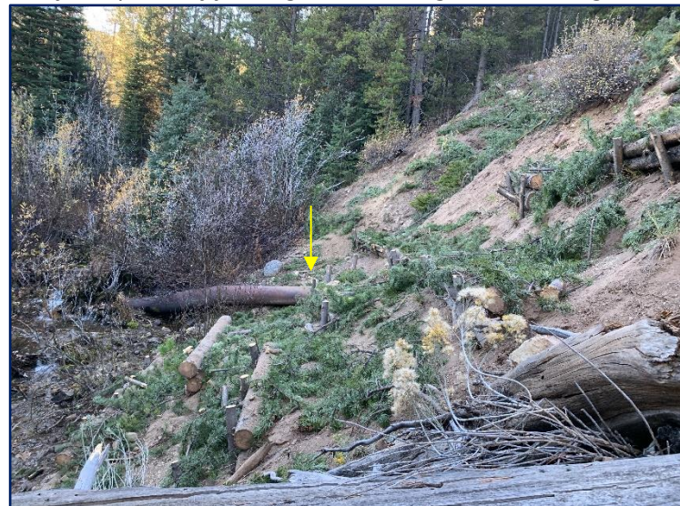
"After" photo of first high and eroding bank post low-tech wattle fence installation. Looking south.
