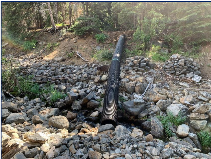
24" x 65' ADS culvert used at the bottom of stream diversion to direct streamflow from the ditch to inside the original channel.
