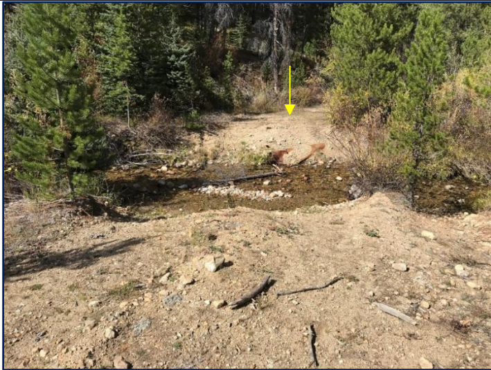
“Before” photo of second eroding bank/stream crossing. Looking west
