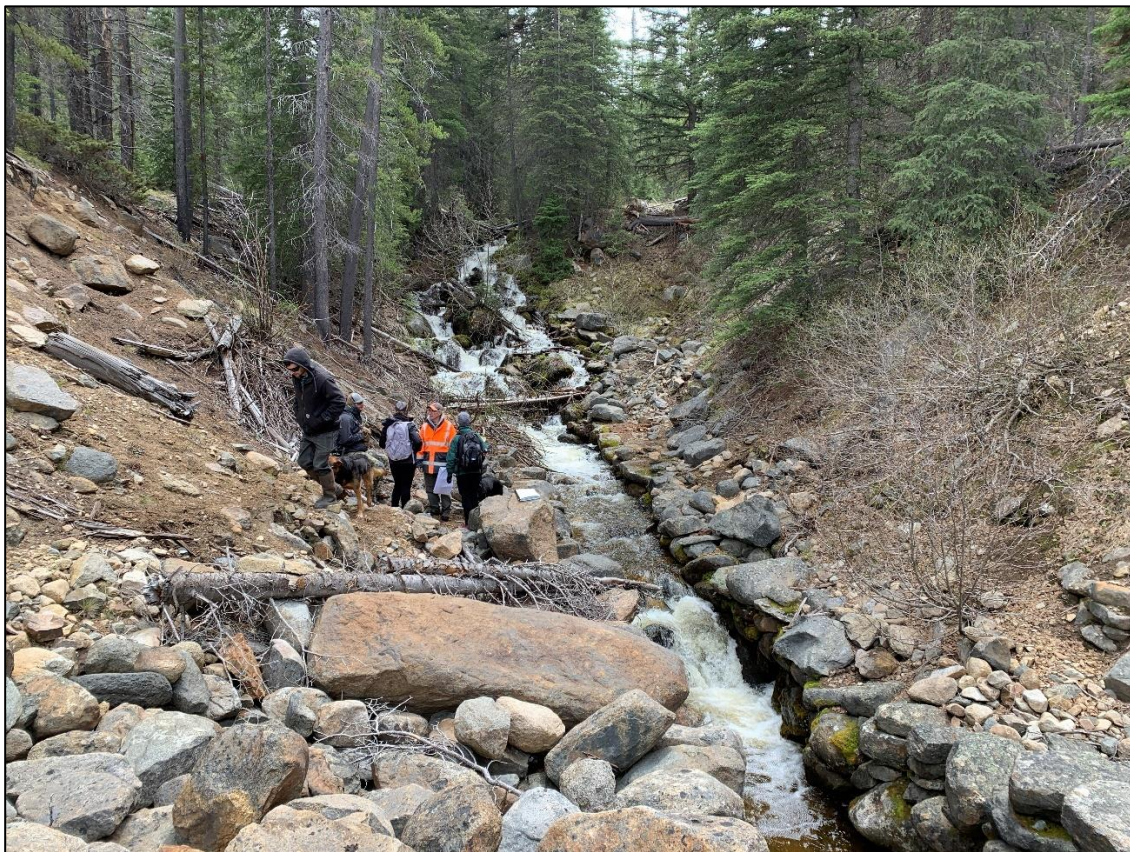
Figure 3. MMI, Watershed Consulting and BHWC at the project site during the June 14, 2021 pre-construction meeting.
