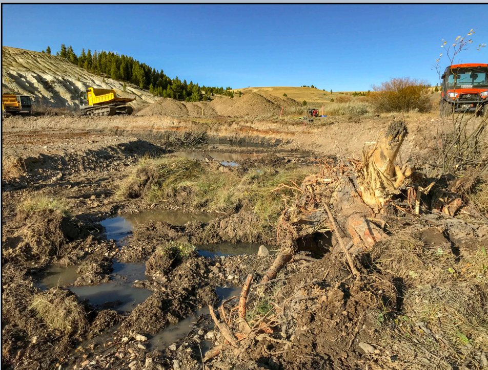
Root wads were strategically placed in the New French Creek stream channel to stabilize and protect stream banks and create fish habitat. Photo by Ben La Porte, Big Hole Watershed Committee.
